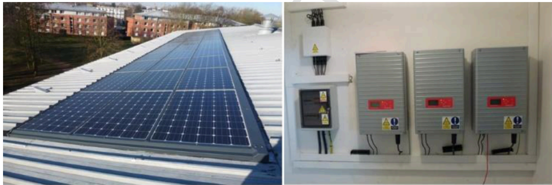
Fig. 12. PV panels installed on the roof of the student residence of Ecole Centrale de Lille and three solar PV inverters.
