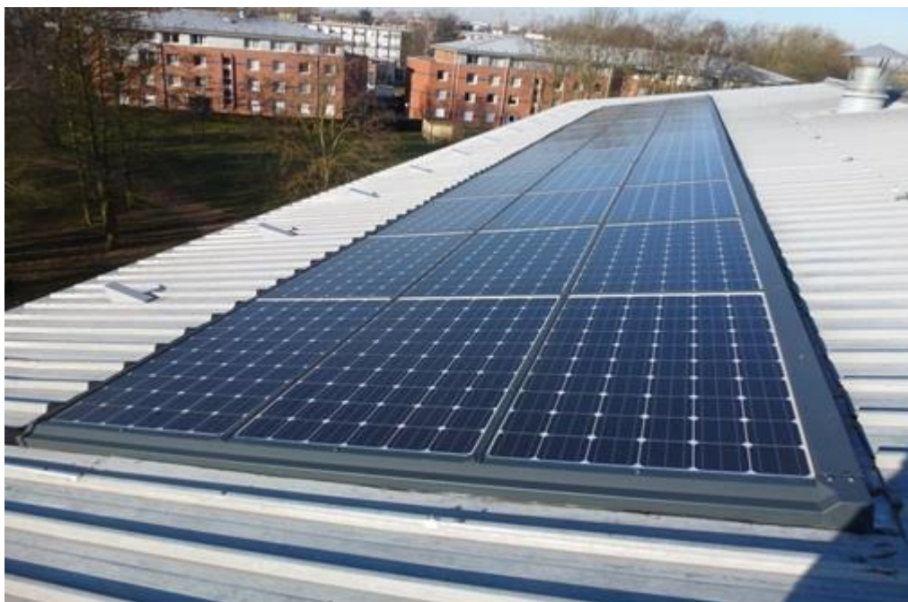
Figure V-10 PV panels installed on the roof of the student residence of Centrale de Lille.
