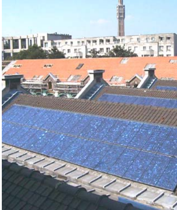
Figure I.18 PV panels at L2EP
