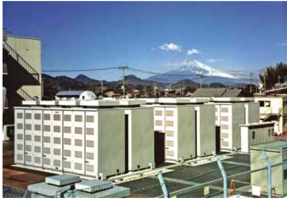
Figure 1.4 NaS battery installation at Tokyo Electric Power Co.'s Ohito (6MW/48 MWh) [www.powermag.com]
